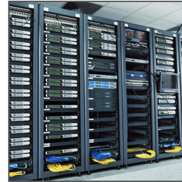
Data Center/Server Trays
